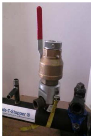
Use view port to confirm the expansion plug is properly seated to stop the flow of gas. Renewal connections or abandonment procedure can now be carried out.
