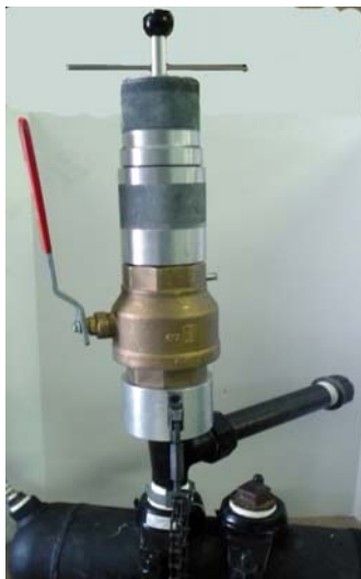
Insert tapered threaded weld plug into main to stop the flow of gas.
