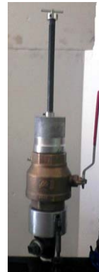
After cap is removed, install expansion plug into throat of tee to stop the flow of gas.
